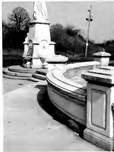
Figure 25: Misalignment of the basin wall (Photograph by author, March 2002)
